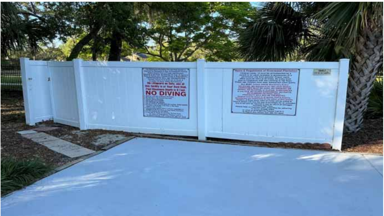
Fence - Pool Equipment
