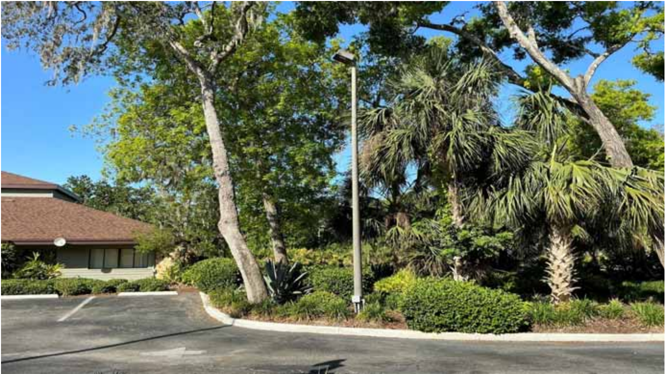
Lighting - Clubhouse Parking Lot
