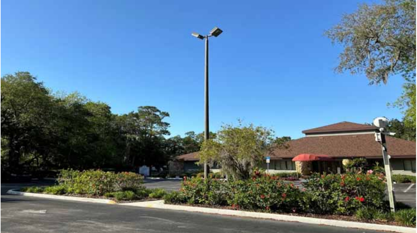
Lighting - Clubhouse Parking Lot
