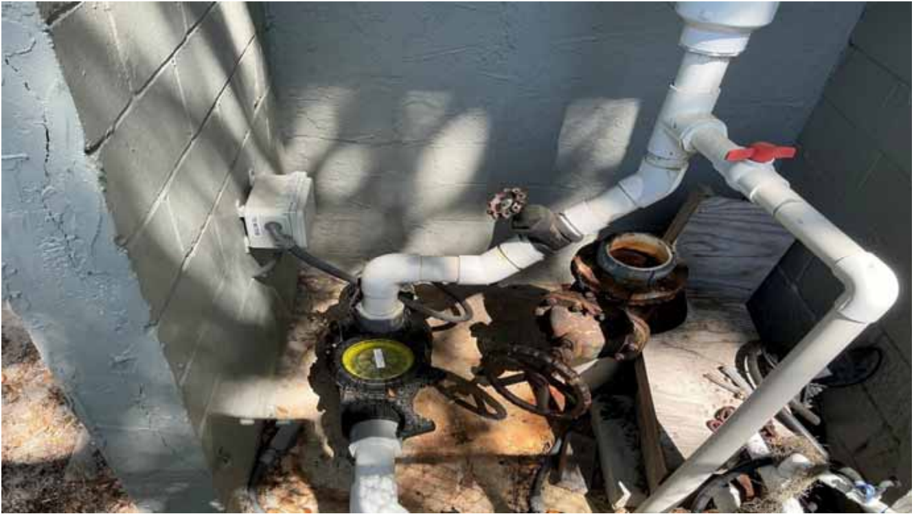
Water Feature Equipment
